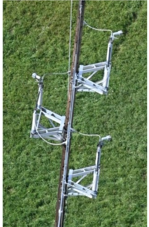
Figure 1. Photo of affected MOAB switch
