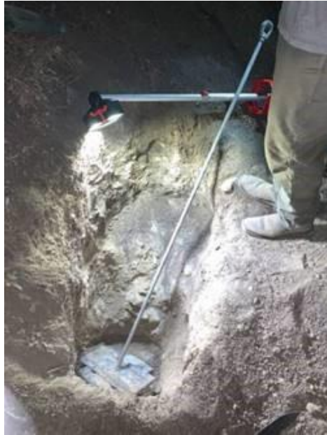
Excavation of PISA anchor directly connected to plate anchor with helix removed
