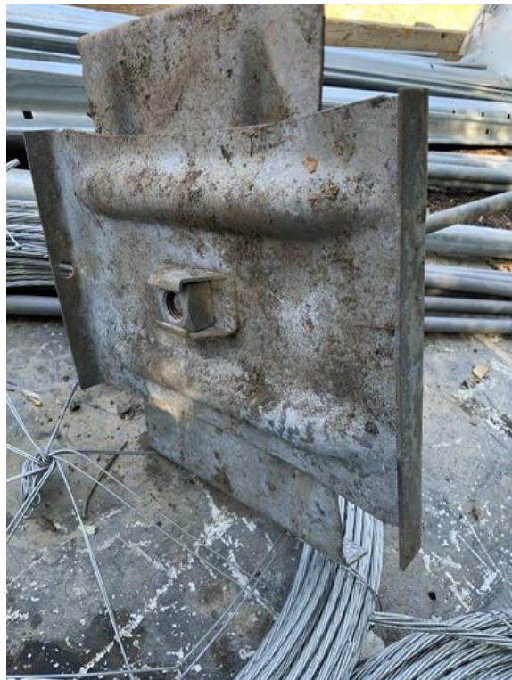
Close-up highlighting the partial threading exhibited in several of the non-conforming PISA installations
