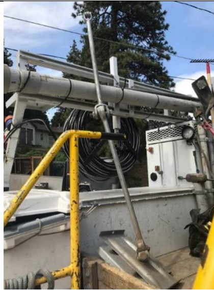
Two 3' extensions daisy chained and connected directly to a plate anchor utilizing an I-bolt
