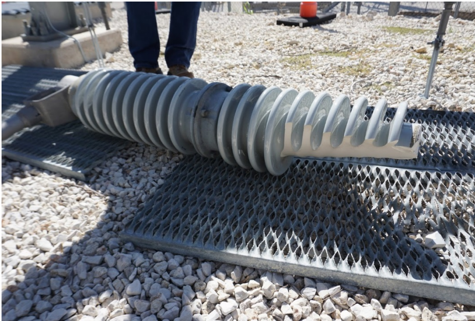
Figure 2. Portion of Failed Insulator and Buss that Fell to Ground
