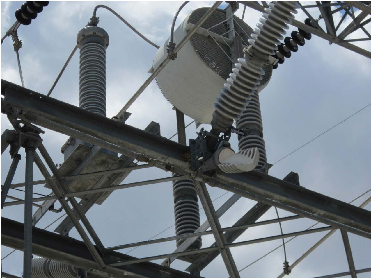
Figure 1. Remainder of Failed Vee Switch
